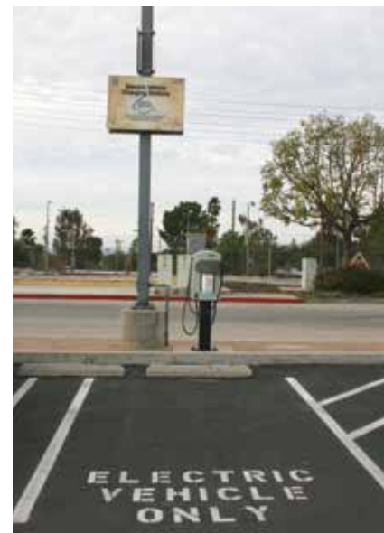
Electric vehicle charging station at the Sylmar/San Fernando Metrolink Station.
