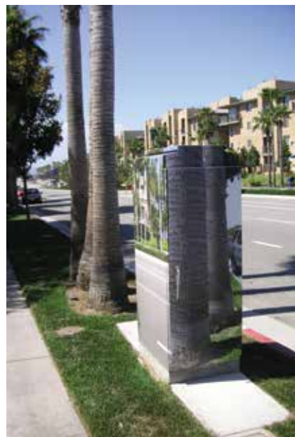
Mechanical equipment can be screened from public view by using innovative techniques.
